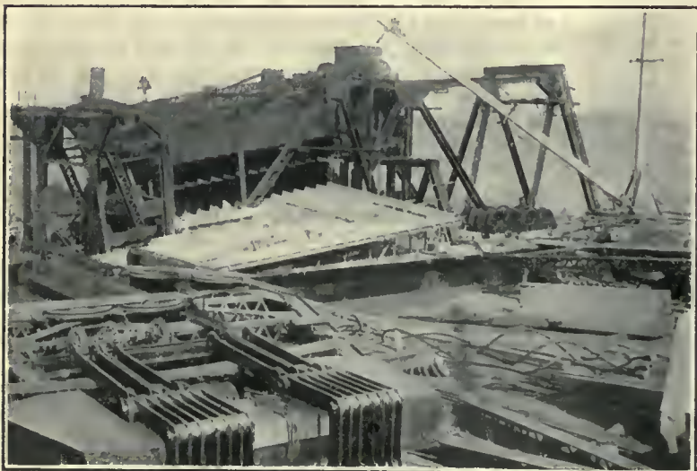
NATOMAS NO. 8 UNDER CONSTRUCTION; SHOWING ARRANGEMENT OF SCREENS AND GOLD-SAVING TABLES; BUILT BY YUDA CONSTRUCTION COMPANY.
